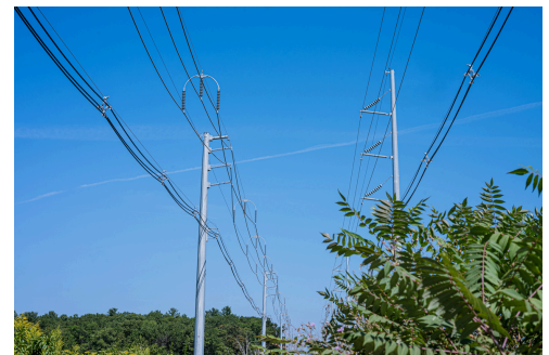
RIGHT-OF-WAY OPTIMIZATION More capacity, same corridor
