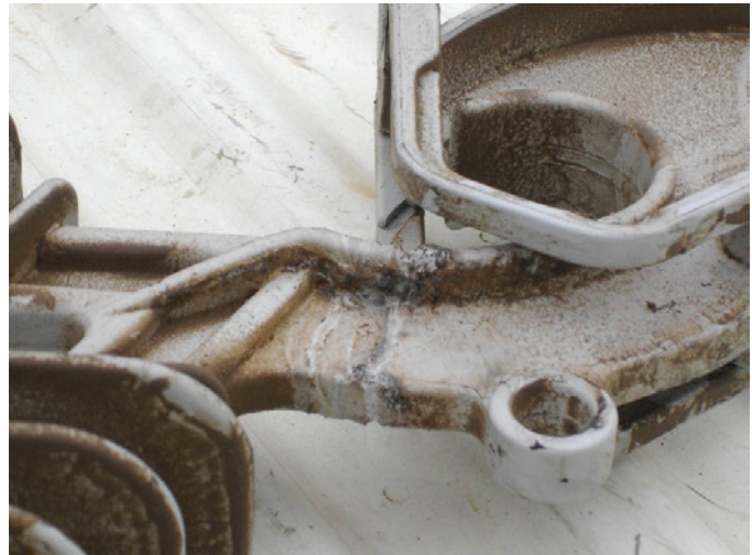
Photo 1: Silica Coated Spacer in Dry, Multiple-Contaminant Environment Exhibiting Dry Band Arcing Prior to Failure
